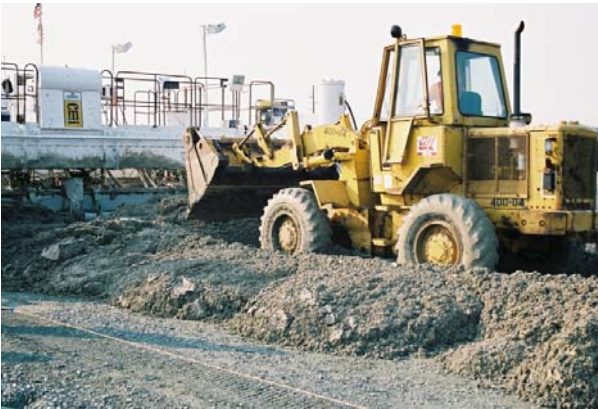
a. Use of end loader is a poor practice.
