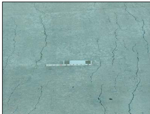
Figure 11.1 – Plastic shrinkage cracking
